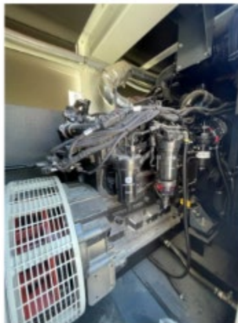
engine connected to generator
