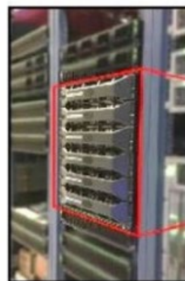
Google GGC Servers
