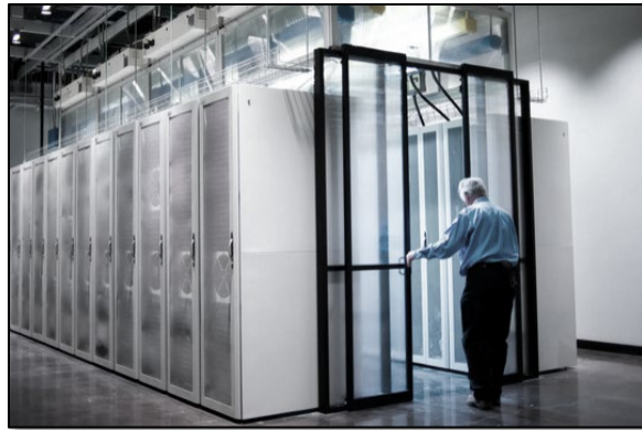
Source: Dave Montgomery, Texas Lures Data Centers, Not for Jobs but for Revenue , N.Y. Times (April 26, 2016) (“a customizable customer pod containing servers at Aligned Data Centers in Plano, Tex.”)
